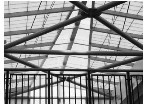
La Jolla Riford Library: Horizontal steel truss at glass atrium and balcony railing.
